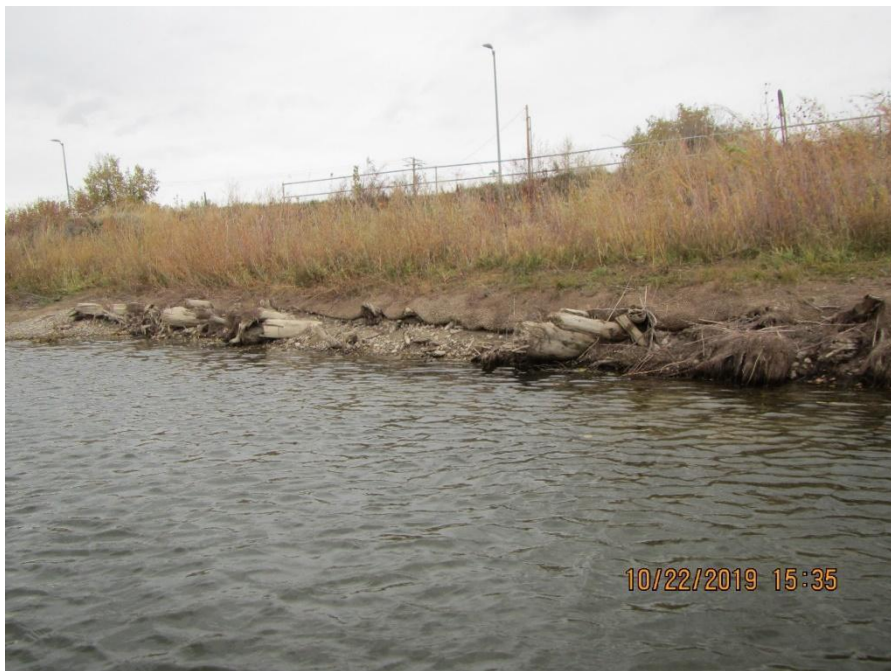
FIGURE A.5.6. Site 2 & 3 - Wyoming Blvd, at the middle of toe wood 3 in-stream, looking at downstream half of toe wood 3.
