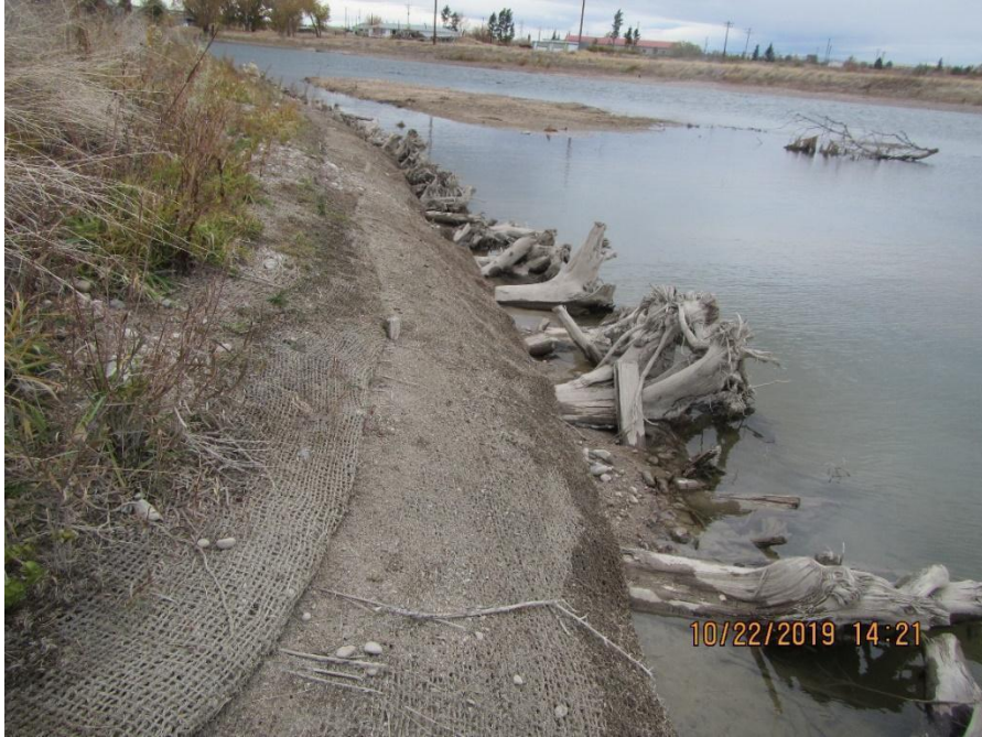
FIGURE A.5.9. Site 2 & 3 - Wyoming Blvd, standing near upstream end of toe wood 5, looking downstream.
